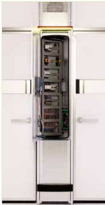
^ Electronics are housed in a sealed enclosure.
